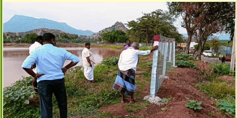
Wire fencing with the help of stones and mesh to avoid encroachment
