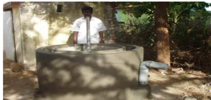
Fixed Model Shakthi Surabhi Bio-Methanation Plant constructed at Kadaladi,Ramanathapuram District.
