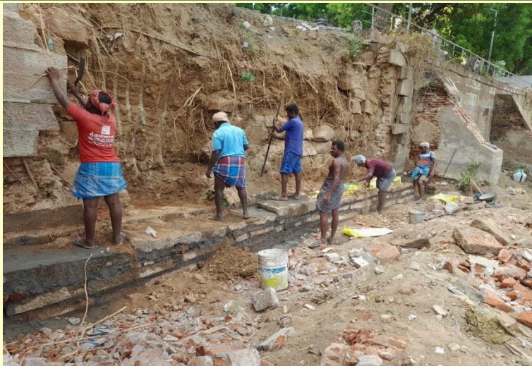
Tree roots have damaged the wall by penetrating inside
