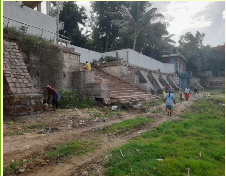
The walls have been damaged because of the roots of the nearby trees entering the wall structure
