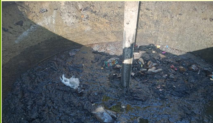
Plant full of sludge
