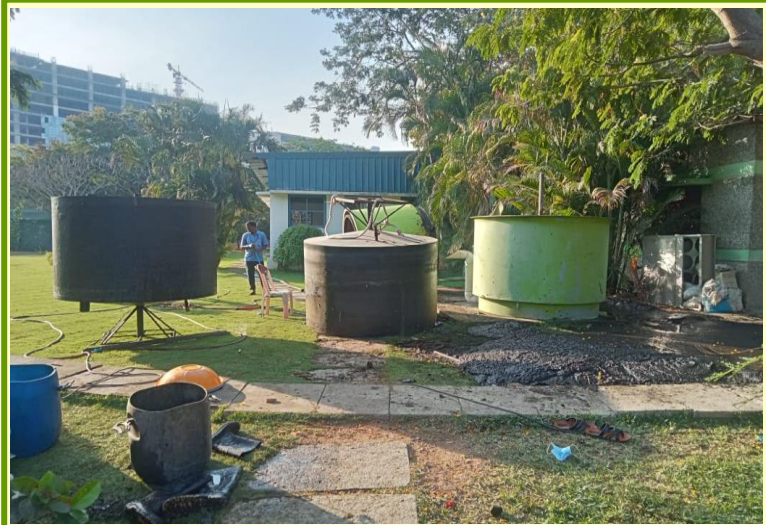
Repairing and touch up work of digester and gas holder is on ...
