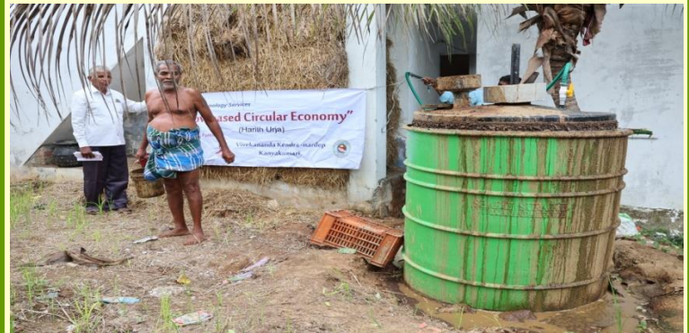
Biogas plant installed - Shri.Subbaih, Kozhikottuppattai
