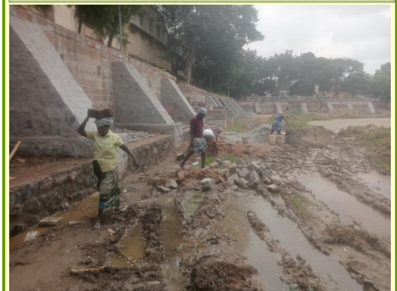
Joining of piers by constructing a parapet wall to strengthen the structure
