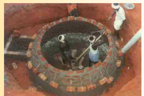
Deenbandhu Biogas plant
